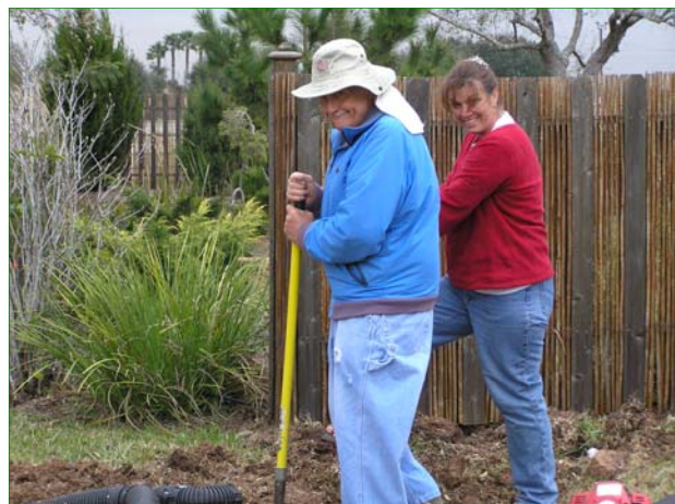
Dell Keene (S04) & Cheryl Huber (S04) working hard fixing the drainage at the Japanese Garden
